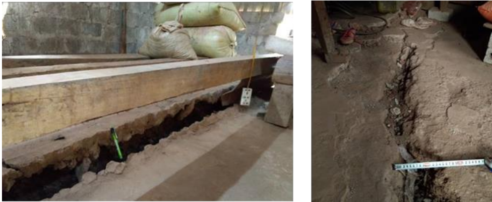
Figure 5. Cracks and subsidence on the foundations of Ms. Sung Thi Pa's house (left) (L3 in Figure 3) and Ms. Giang Thi Chu's house (right) (L4 in Figure 3).
